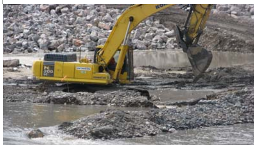
Coffer dam is breached! Clark Fork and Blackfoot Rivers begin to flow into the new channel.
