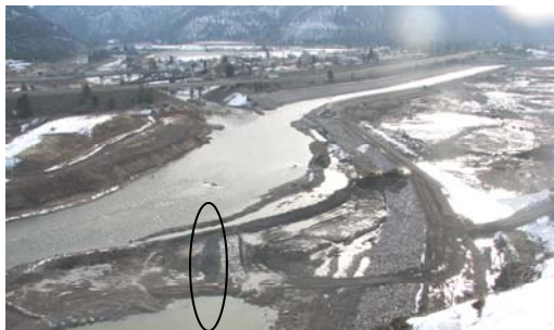
9 am: Pre-breach view of the project area. Oval shows area where coffer dam will be breached.
