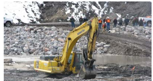
2 pm: Removing material to begin the breach of the spillway coffer dam and divert the Clark Fork and Blackfoot Rivers into the new channel
